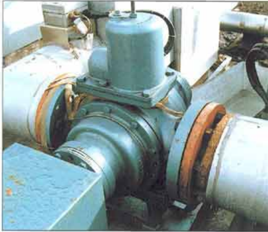
G2000 Pump with Heat Tracing prior to lagging.
